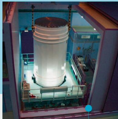
TRANSFER OF A CASK TO THE HIGH-LEVEL WASTE STORAGE BUILDING
