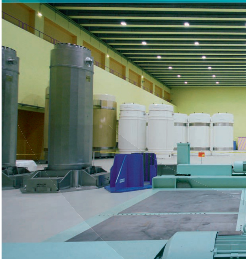
VIEW INTO THE CASK STORAGE HALL
